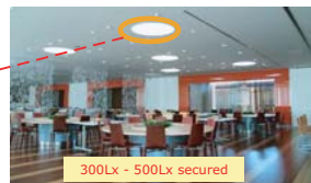
300Lx - 500Lx secured light emitting part of light duct in dining hall
